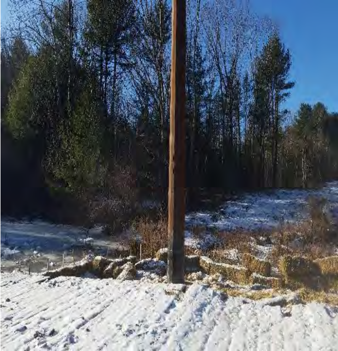
Fig 5: Str. 102. Viewing southwest in wetland NW6. (01-17-20). Straw bales have since been staked in.
